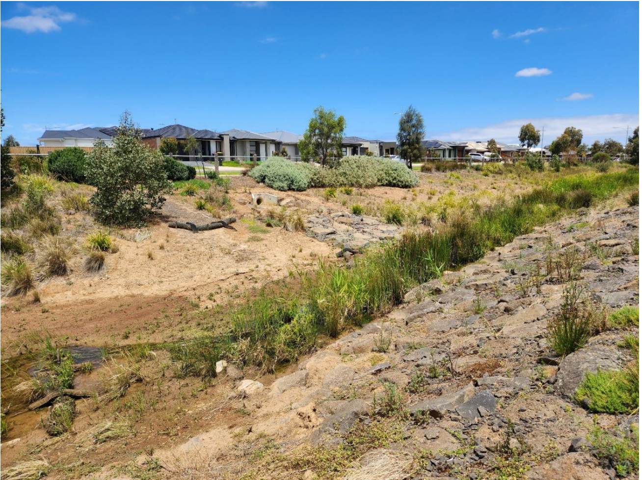
Photo 2 Western extend of Wetland 1 near Farm Road, showing areas of bare ground and sediment control. Photo taken on 16 December 2025, facing approximately south-west.
