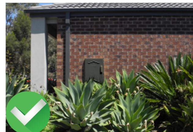
Example of meter box on side of house screened by planting and painted to match the downpipe and house.
