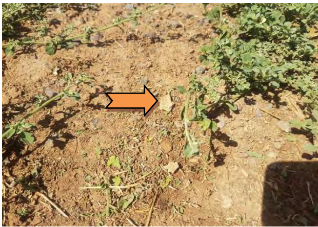
Photo 1. Asbestos-containing fibre cement sheet debris located on the soil surface within Riverwalk Stage 16.
