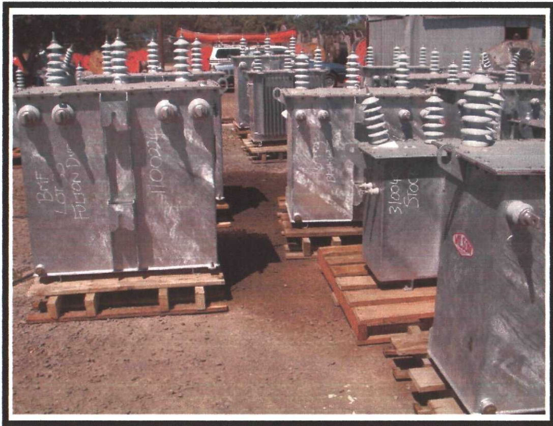
Photograph 1 – Oil staining in the transformer storage area.
