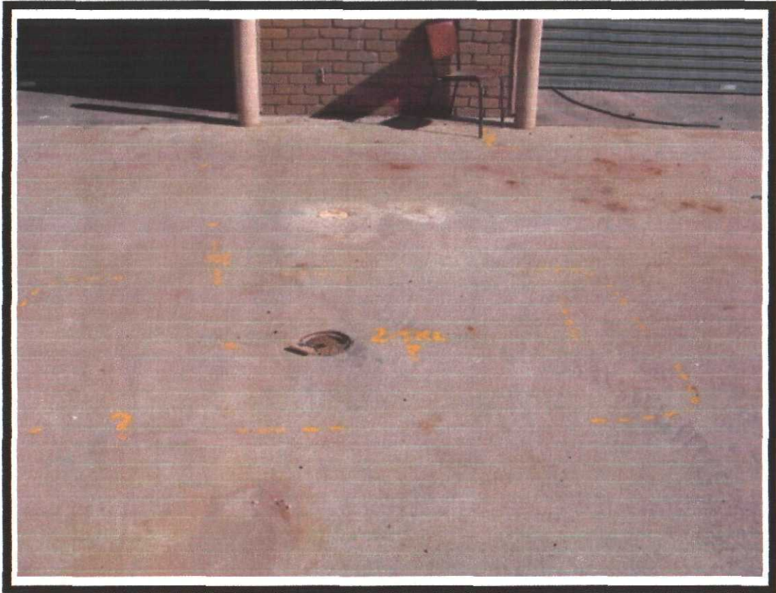
Photograph 3 – Waste oil UST located to the north of the workshop.
